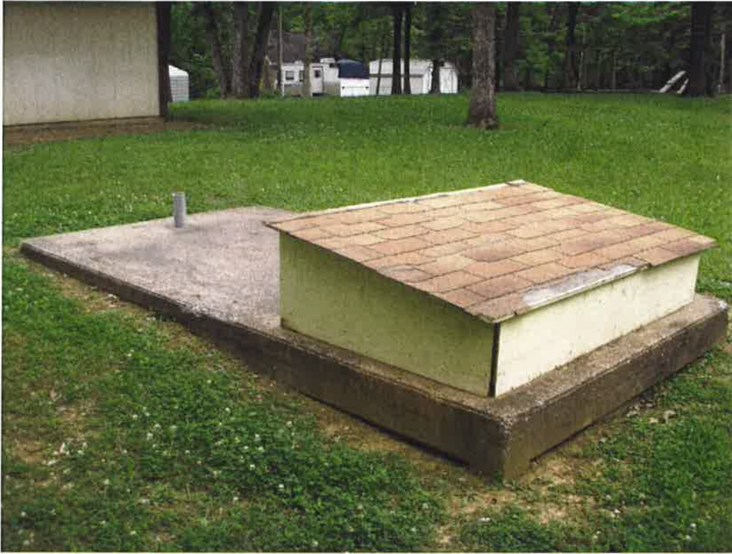
Existing Lift Station at Comfort Station
