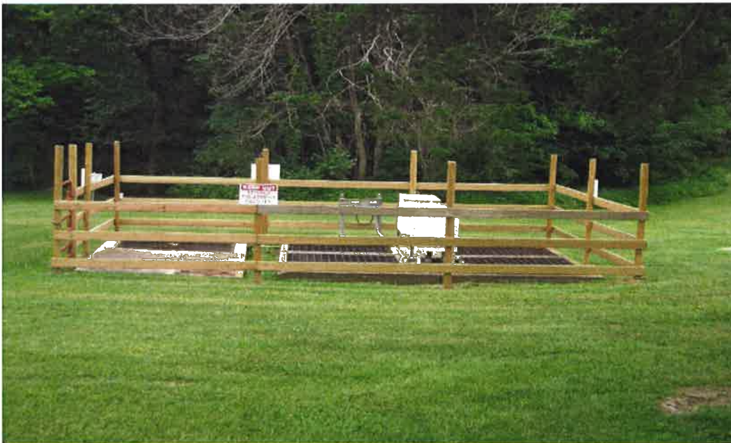
Existing Mechanical Treatment Plant- Outfall #2
