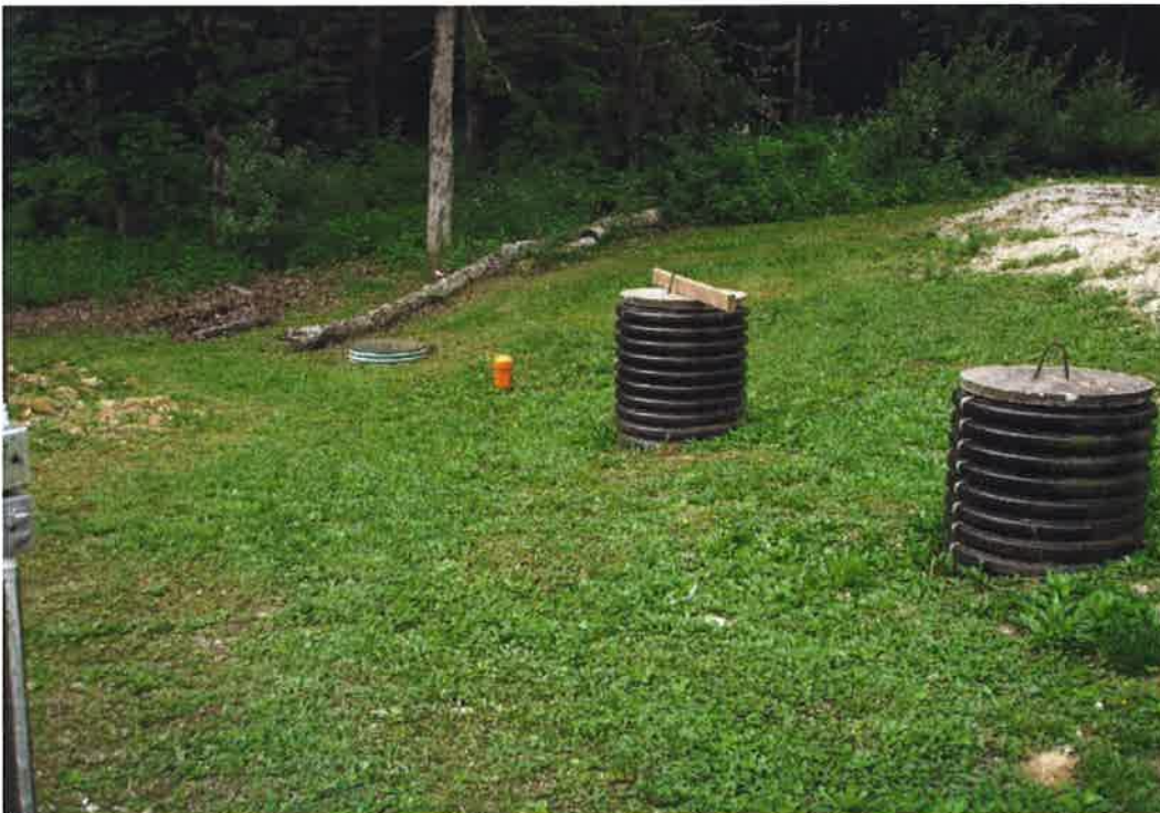
Existing Lift Station
